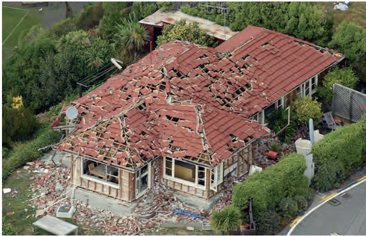
Fig. 1.3 severe damage to a single family house in Light-Weight Timber Construction with non-bearing masonry between the frames and 'heavy' roofing [32]
